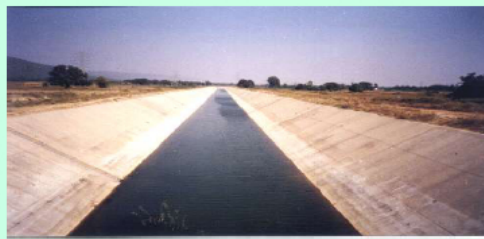
Common Water Carrier at 13.71 km
